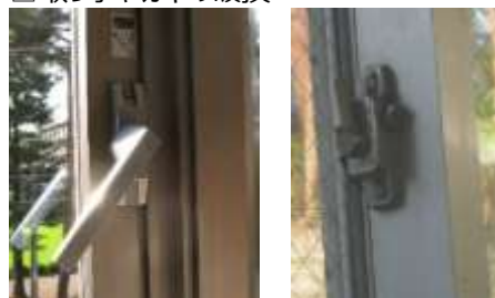
取っ手やカギの破損
