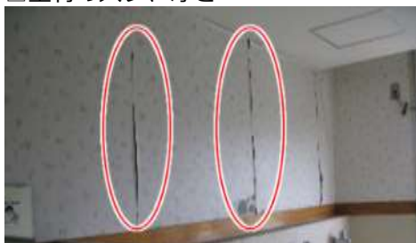
□壁材のズレ、浮き
